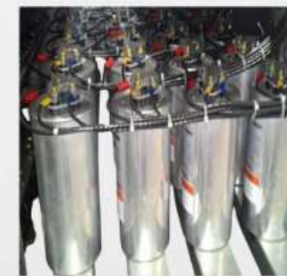
Capacitor Bank/ Detuned Capacitor Bank
