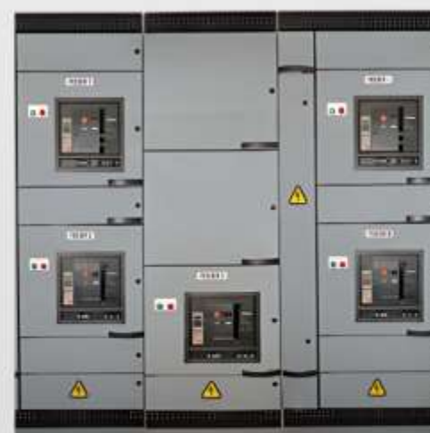
Low Voltage Switchgear
