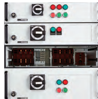
IP2x shielding of the vertical busbar
